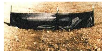
Figure 9. Poor installation, water can flow around the ends causing additional erosion
