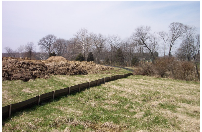
Figure 1. A silt fence at the perimeter of a construction site. Photo Credit: USEPA/Wikimedia
