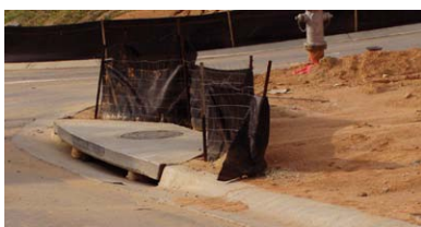
Figure 7. This silt fence doesn't work
