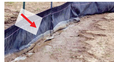
Figure 16. Poor compaction has resulted in infiltration and water flowing under this silt fence causing retained sediment washout.
