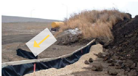
Figure 17. Back of silt fence on part of the stockpile's perimeter.
